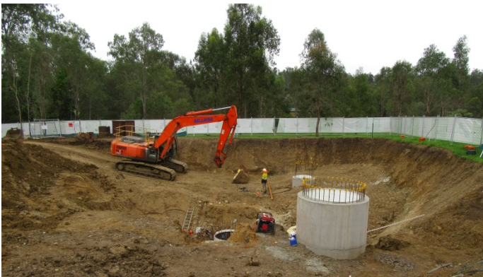
Excavation and new maintenance holes at the Ferny Gully SPS site (Oct 2018).
