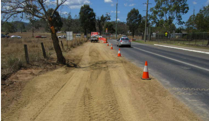
Site of rising main installation, opposite Fernvale State School on Forest Hill Fernvale Road (October 2018).
