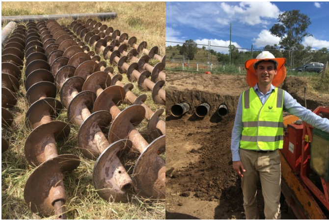
Left: Augers used to drill out the earth to make way for the pipe. Right: Casing pipes installed under Forest Hill Fernvale Road and Project Manager, Jonathan Farrell, with the thrust bore machine (Nov 2019).
