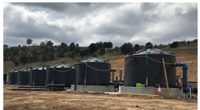
New service water tanks installed at the Lowood STP (Jan 2019)
