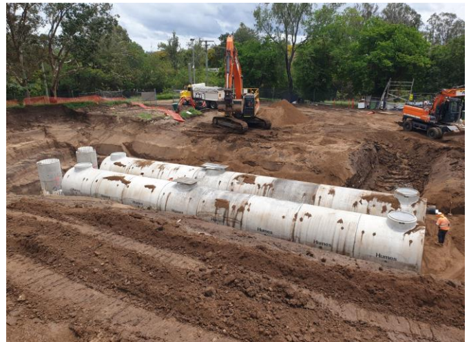
Image – Lowood STP Demolition site and the new underground storage facility for the new Lowood PS (Jan 2022)
