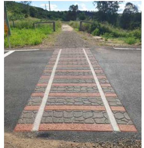
Image – Rail Trail stencil painted at the crossing of the driveway of the new STP
