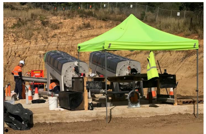
Above: Cube presses being installed. These will be housed in the sludge dewatering building and will compact solids and extract liquids (July 2019).
